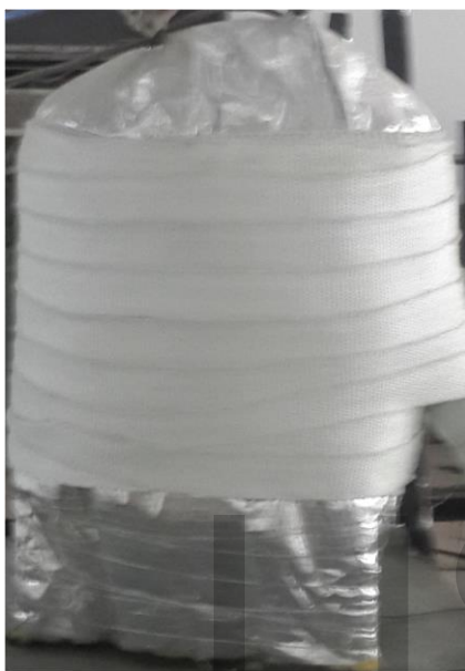
Fig. 4. Heat storage tank
